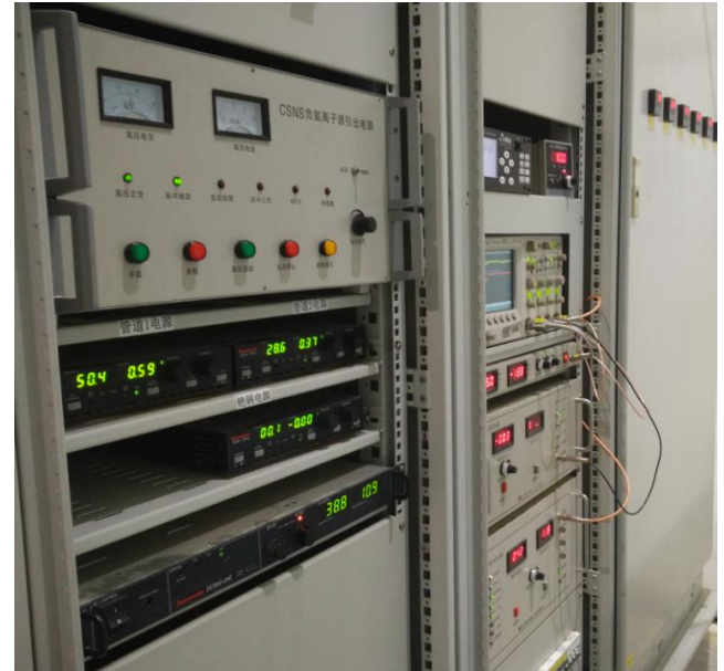
Local control platform
