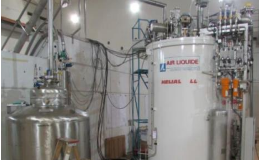
G. Hodgson et al., Acceptance Tests and Commissioning of the ARIEL e-Linac Helium Cryoplant, Cryogenics 2014 (IIR)
