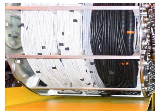
View of a cable chain (RJ45 connection between FE and VFE)
