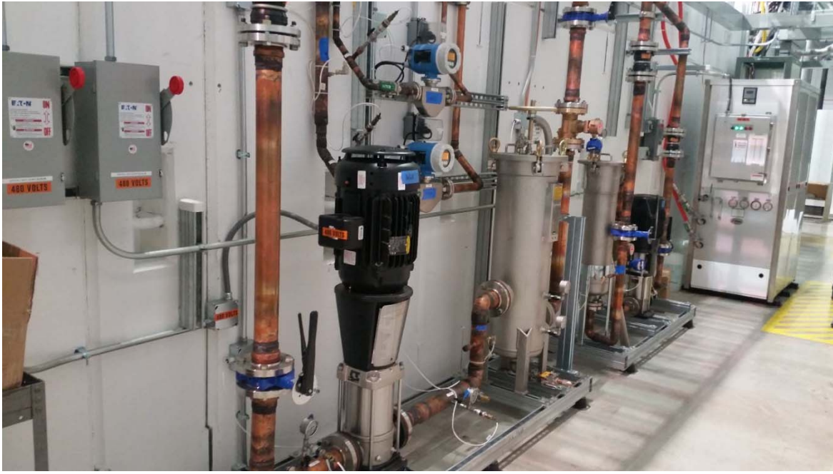
Figure 4.7: RFQ LCW showing separate Vane and Wall LCW skids. These skids incorporate pumps, filtration, and precision flow measurement.
