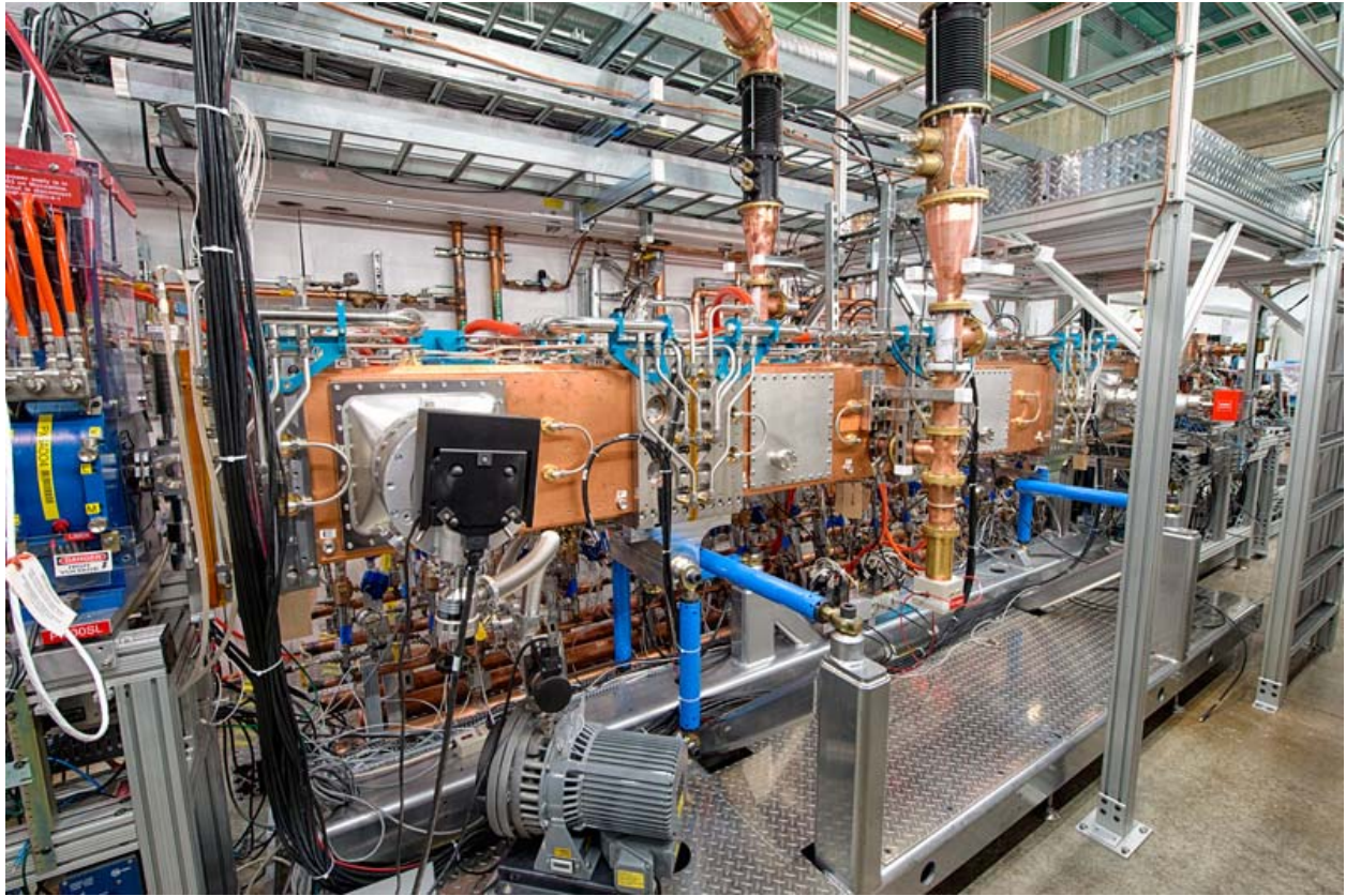
Figure 3.7: RFQ installed in PIP2IT beamline.
