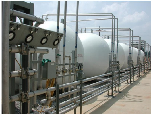
Figure 7-13. Gaseous helium storage vessels at JLAB
