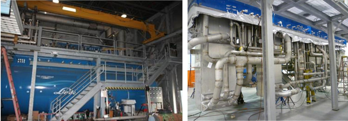
Figure 7-9. Two views of the lower 4.5K cold box section and internal piping installed at JLAB
