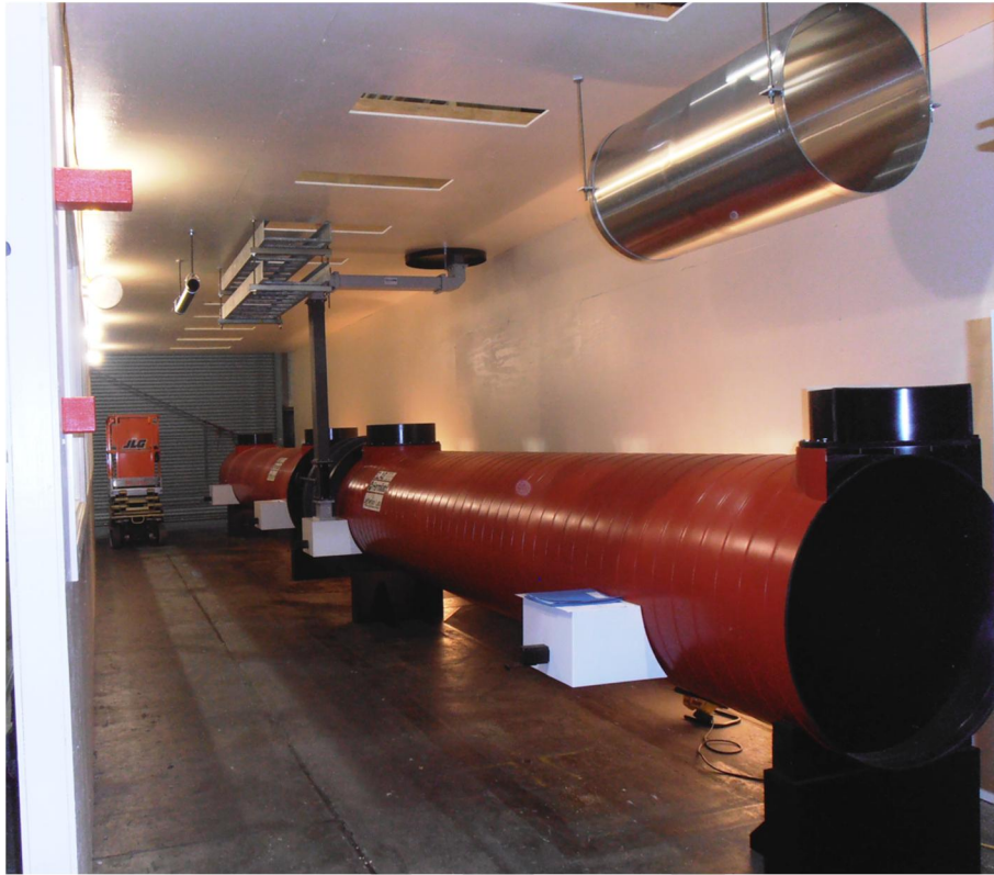
Figure 4-9. SLAC tunnel mock-up with cryomodule, couplers, cryo-distribution and racks to understand installation issues.
