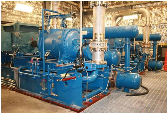
Figure 7-5. Warm recirculation compressors at JLAB
