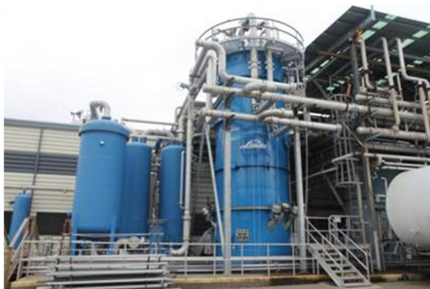
Figure 7-8. Upper temperature 4.5K cold box at JLAB (on right)
