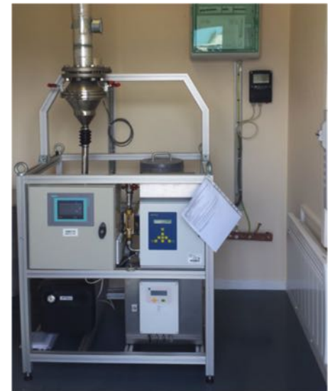
Ventilation monitoring CERN/SAPHYMO
