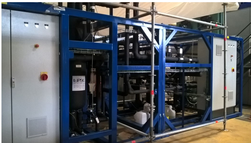
Figure 11.5: CO 2 cooling plant demonstrator located in Building 180 at CERN.
