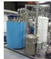
2012 2kW@20K helium refrigerator
