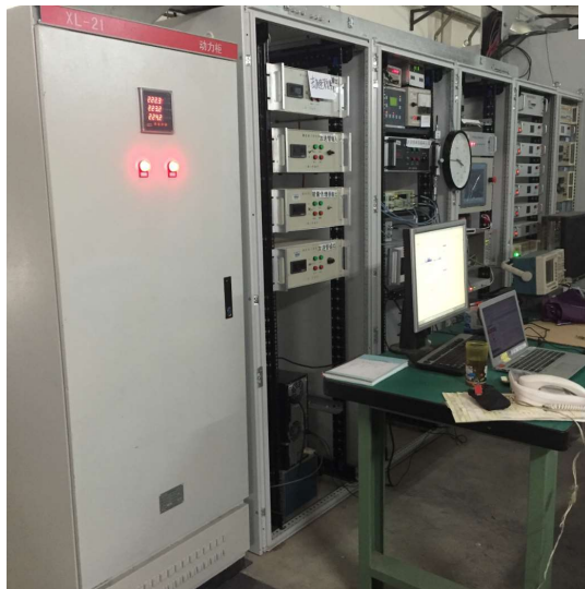
Modulator and klystron
