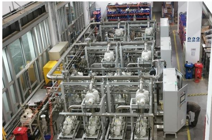
Cryogenic system hall in Jan. 16, 2020
