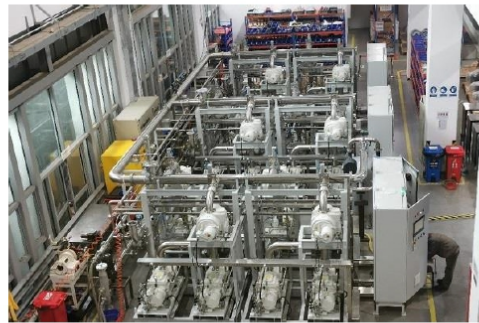
Cryogenic system hall in Jan. 16, 2020
