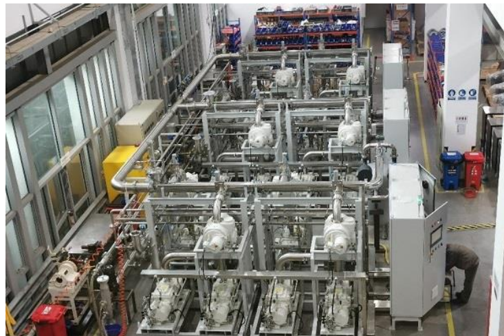
Cryogenic system hall in Jan. 16, 2020
