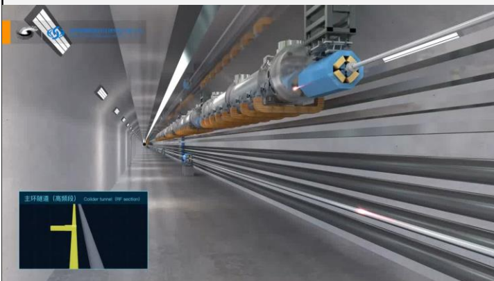
Collider ring tunnel (RF)
