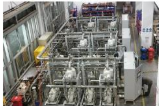
Cryogenic system hall in Jan. 16, 2020
