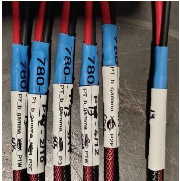
LV cables一处标签
