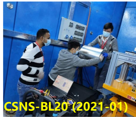
Install in the Beamline
