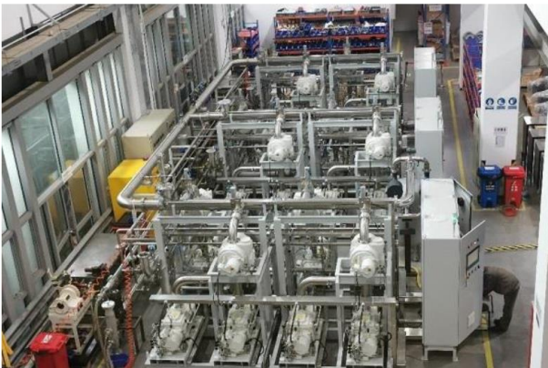
Cryogenic system hall
