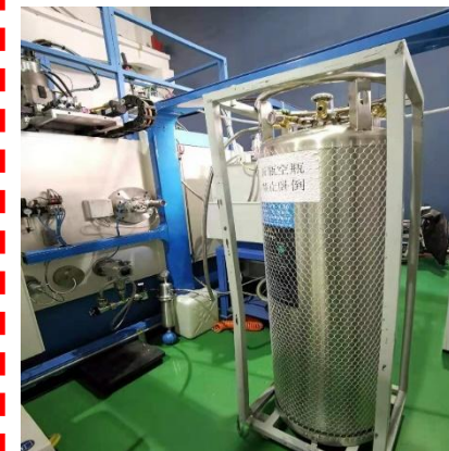
N2 Cooling system
