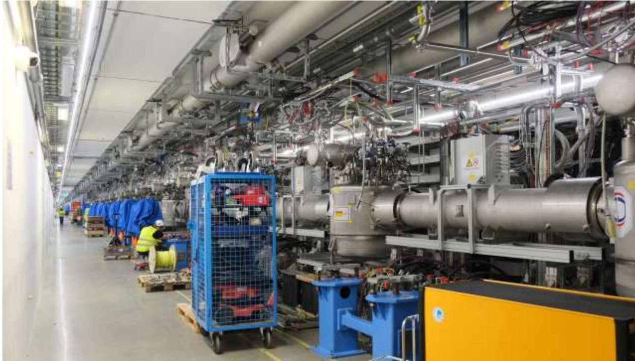
Cryo Systems for superconducting linac components Cooldown of the Cryogenics Distribution System (CDS)
