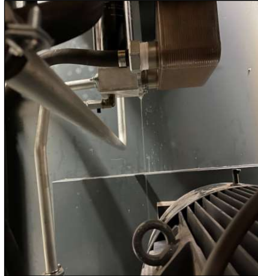
A leak on the compressor heat exchanger
