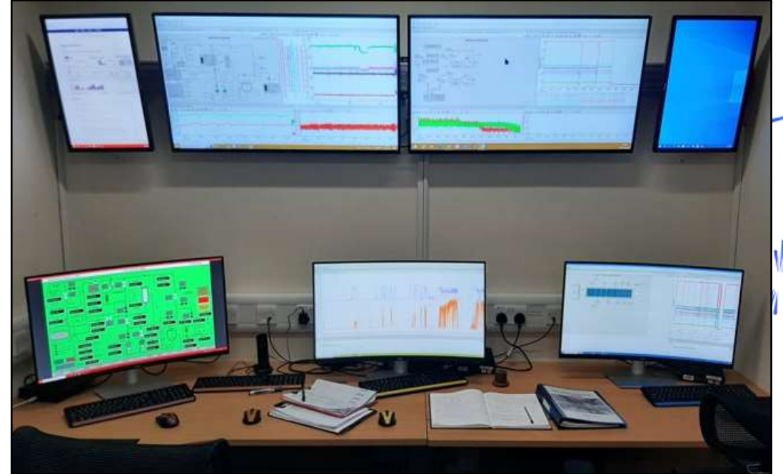
TS1 Target control room computer screens
