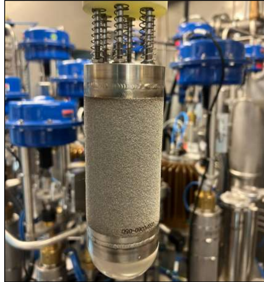
A photo of the methane system filter unit
