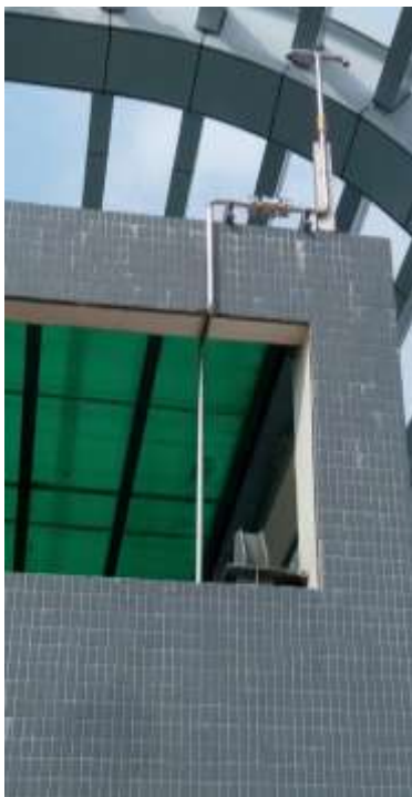
Part of hydrogen vent line
