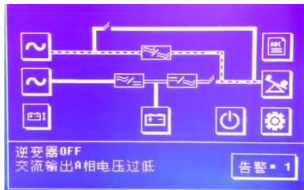
UPS switched to bypass
