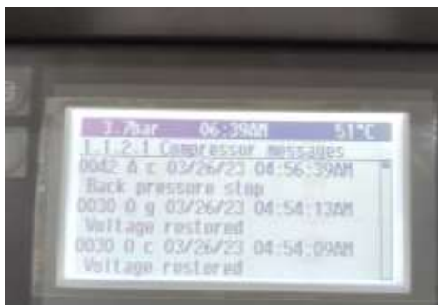
Compressor voltage restored
