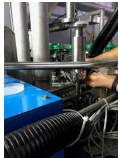
Replace bursting disc
