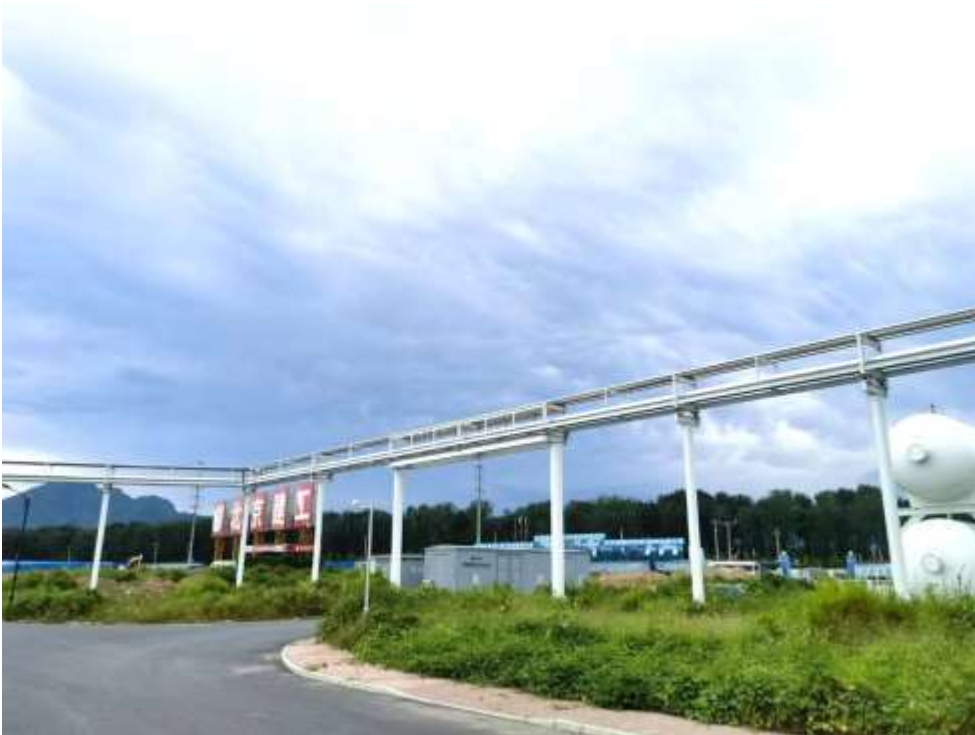
Transport line from cryogenic hall to HEPS
