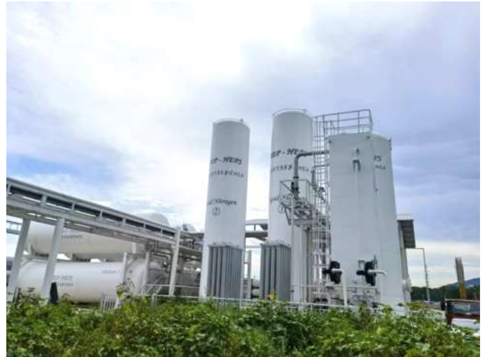
Tank area and cryogenic hall
