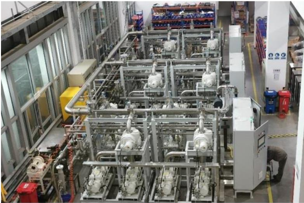
Cryogenic system hall
