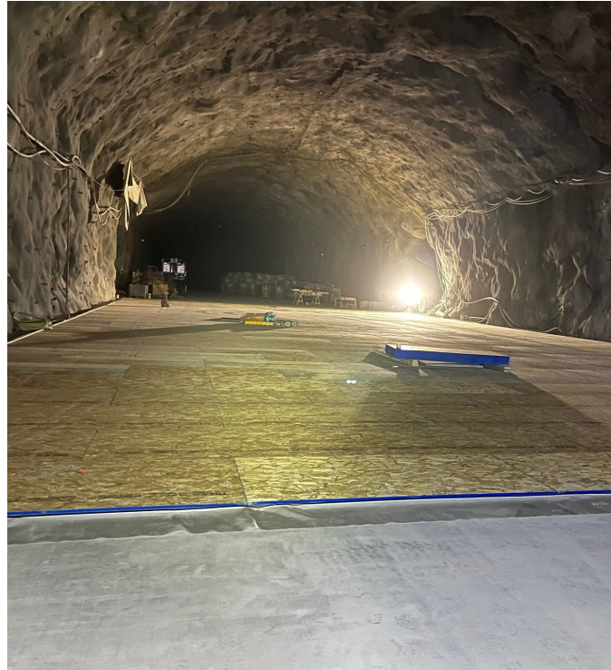
Central Utility Cavern
