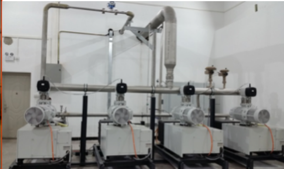
2K pumping system
