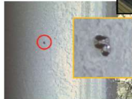
Figure 1: A defect observed with inspection camera.
