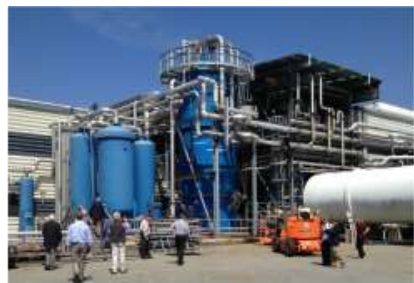
Large cryogenic plant
