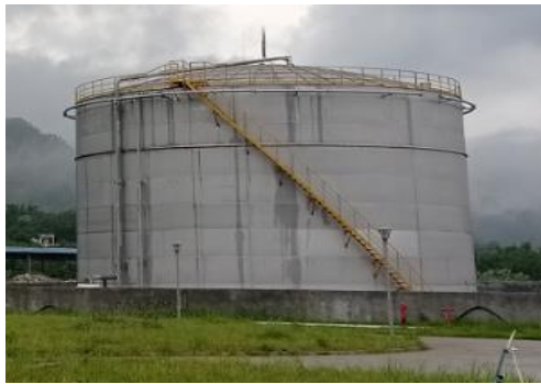
5000 m 3 LAB storage tank
