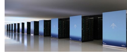
Fugaku supercomputer (440 PFlops)
