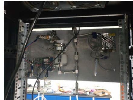
Front and back panel of the updated leak test system
