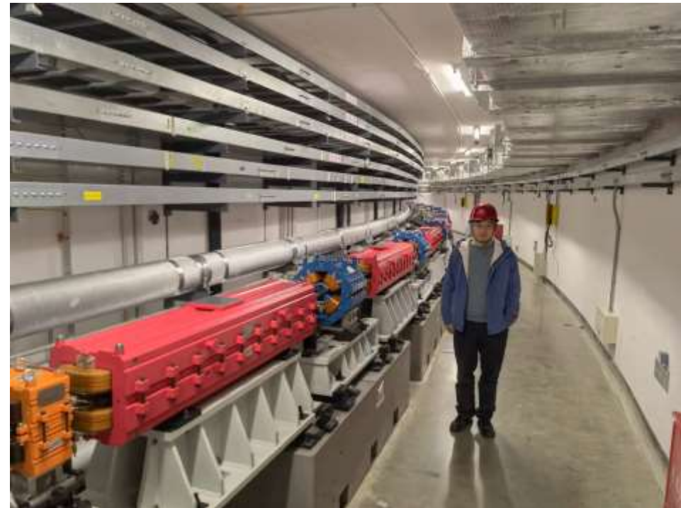
The HEPS Booster magnets in tunnel
