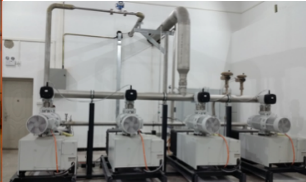
2K pumping system
