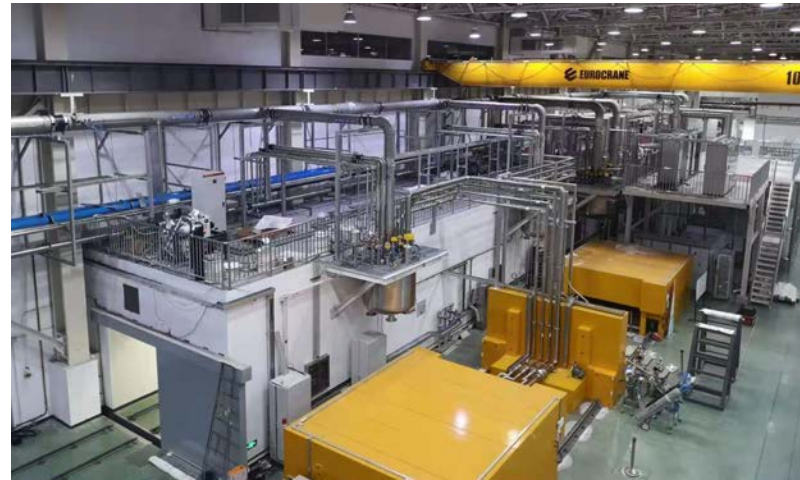
Cryogenic distribution in No.1 test hall
