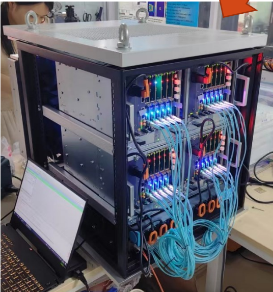
To be upgrade with internal switch
