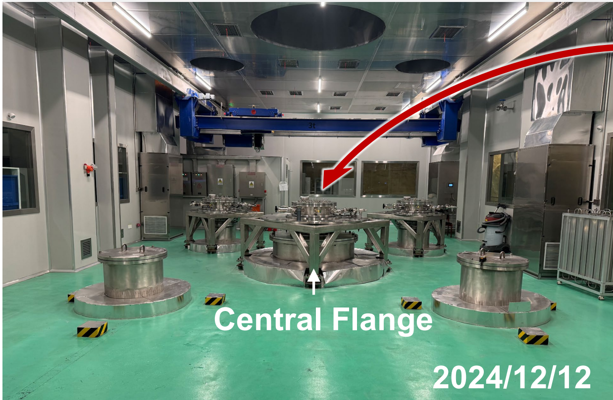
Top Clean Room
