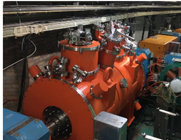
3W1 in BEPCII tunnel
