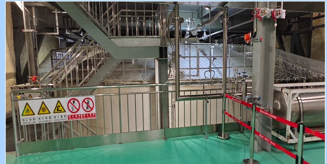
Top of the commissioned LN 2 tank
