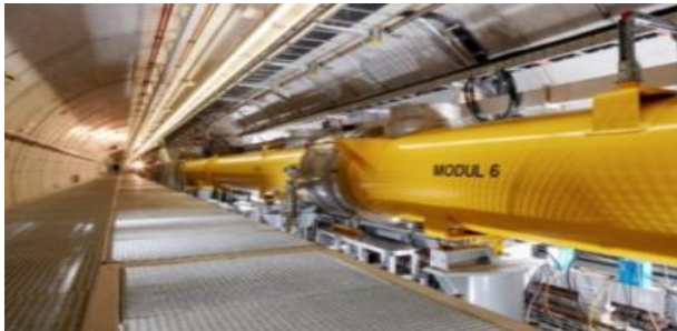
TESLA type superconducting accelerating modules 1.3 GHz
