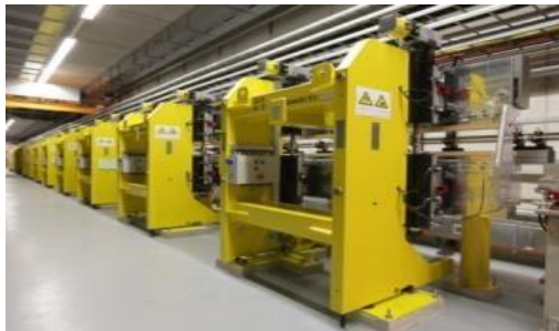
FLASH2 variable gap undulators
