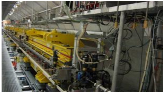
FLASH1 fixed gap undulators
