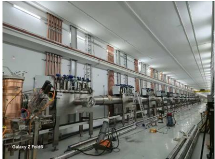
The RF power transmission line
