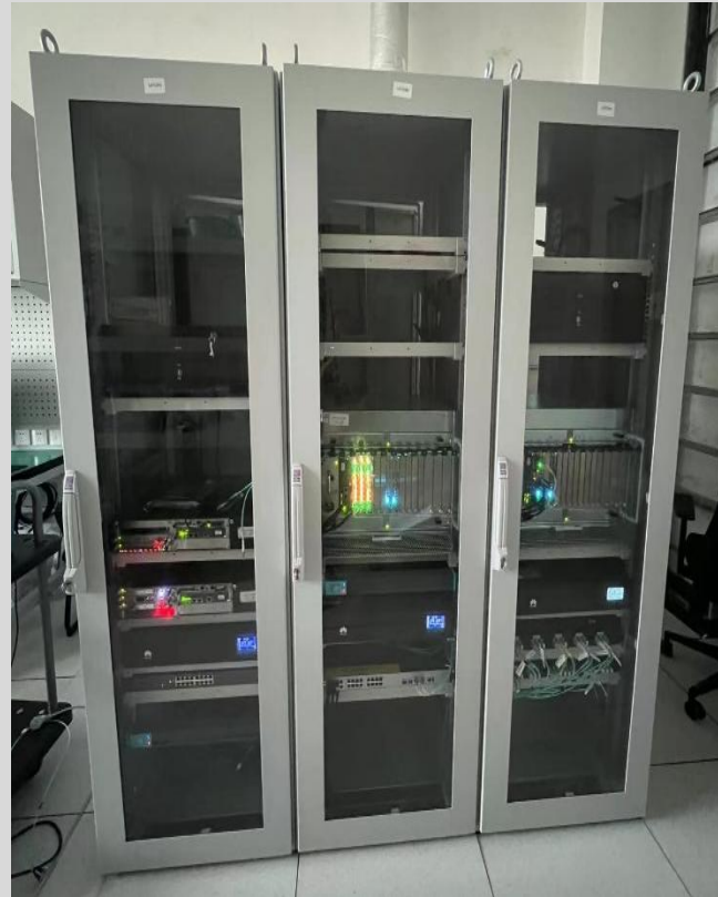
1. Temporary Main Timing Station 2. Microwave and Power Source Timing Station
