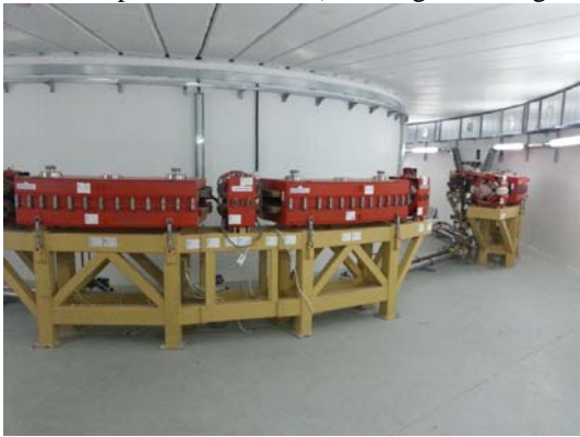
Figure 13: Booster Girder with Magnets inside tunnel
