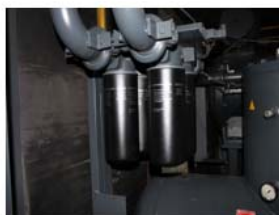
Replace oil filter
