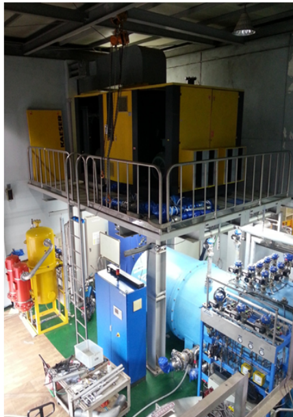
1 kW Helium Refrigeration
