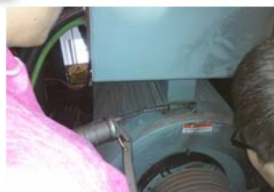
Grease injection in bearing
