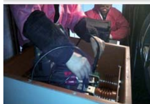
Electric resistance inspection
