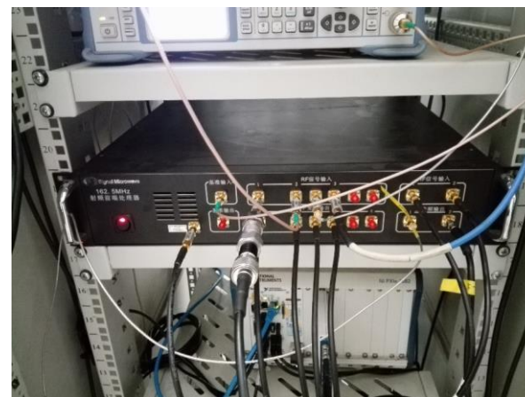
RFQ LLRF control system
