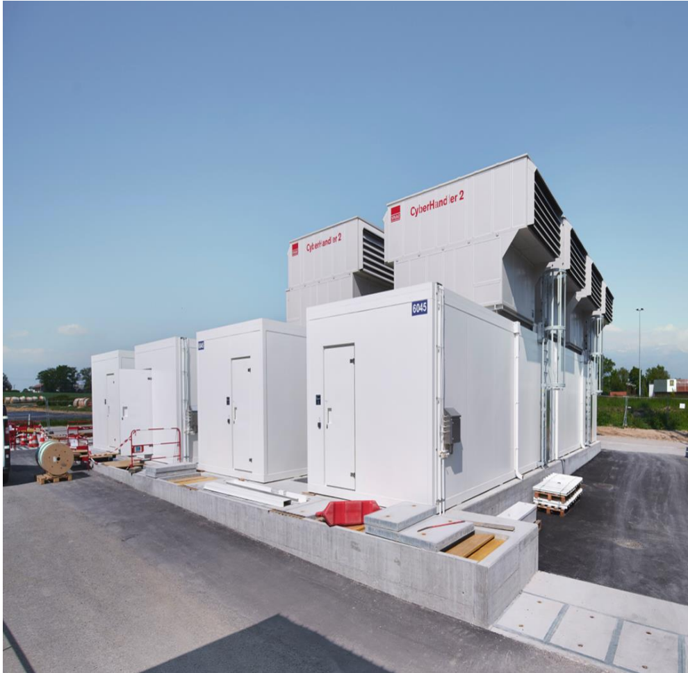
Total 6 modules: 2 already running, 2 under commissioning, 2 delivered.
