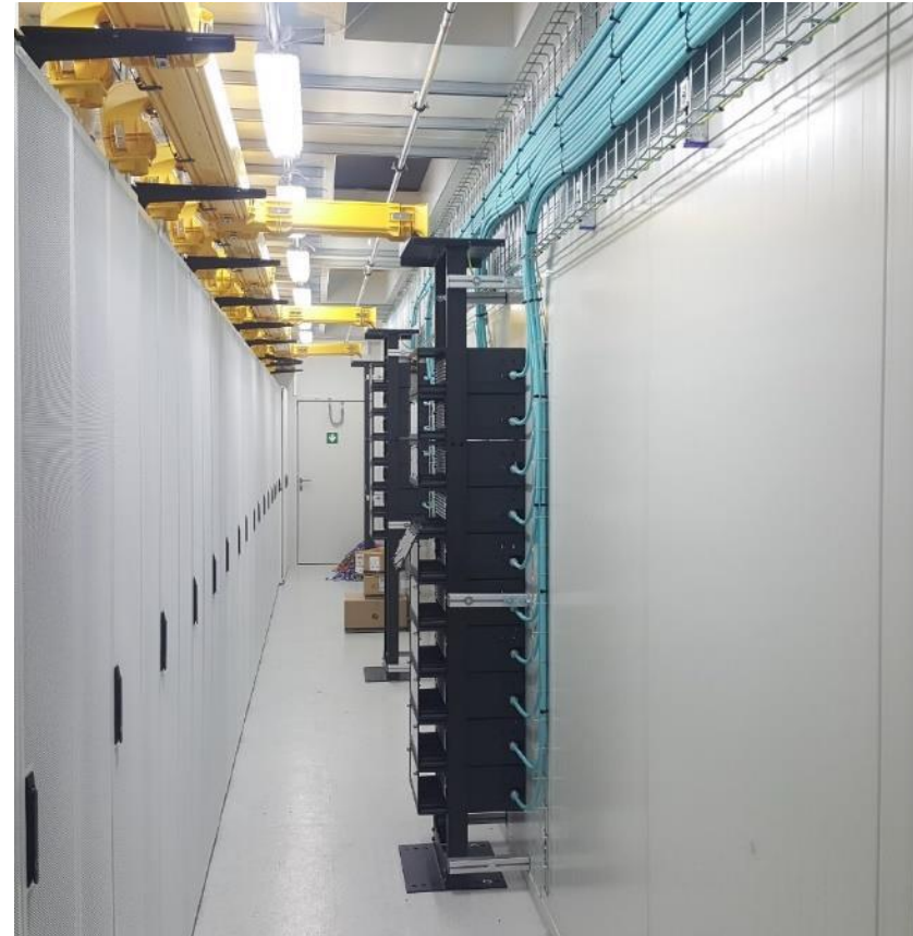
All long optical fiber trunks between FE & the data center are pulled, connected and tested (# ~19,000)
